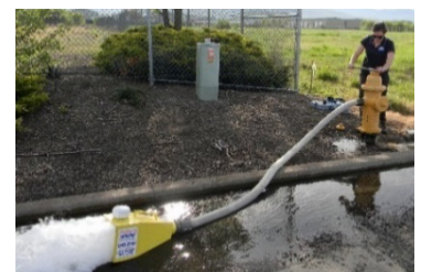
Routine maintenance such as hydrant operation and flushing helps ensure water quality from the source to your tap.
