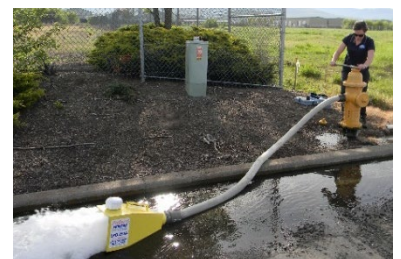
Routine maintenance such as valve turning and hydrant flushing helps ensure water quality from the source to your tap
