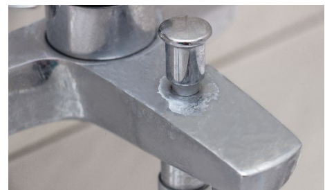
Mineral scale on water faucet
